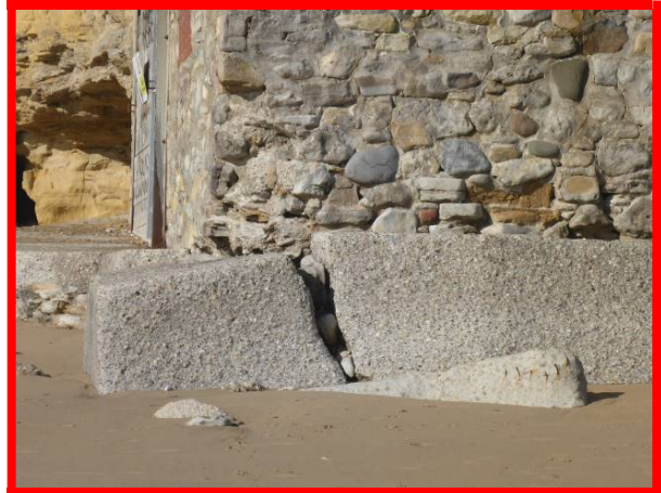
Undermining and cracking at storage building on south face of buttress to access steps (/0401C01)
