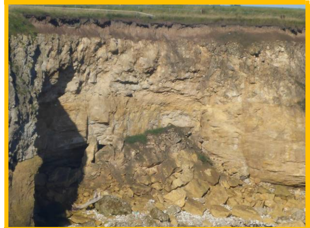
Residual debris from previous large rock fall in Frenchman's Bay (/0401C04)
