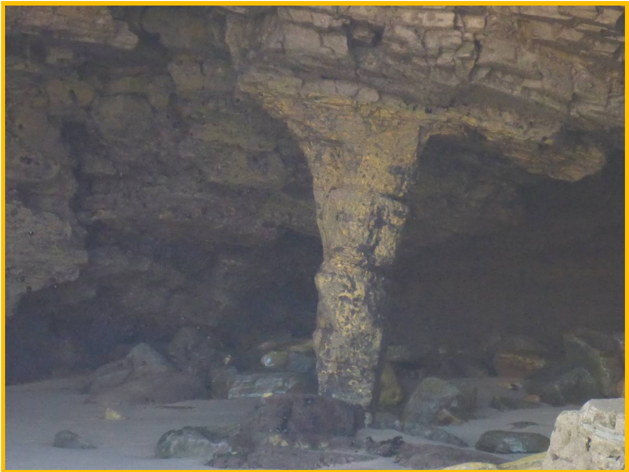
Thin rock column within cave along toe of Marsden Rock (/0401C03)
