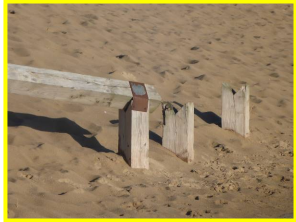
Missing timber fence rail at access point (/0201C01)
