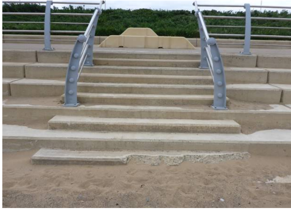
Damaged beach access step at northern end of promenade in need of repair when seen in 2018 (/0102C02)
