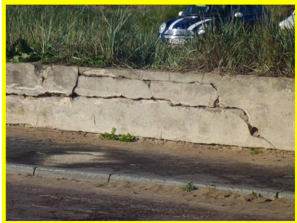
Cracking to render on wall at rear of promenade (/0202C05)
