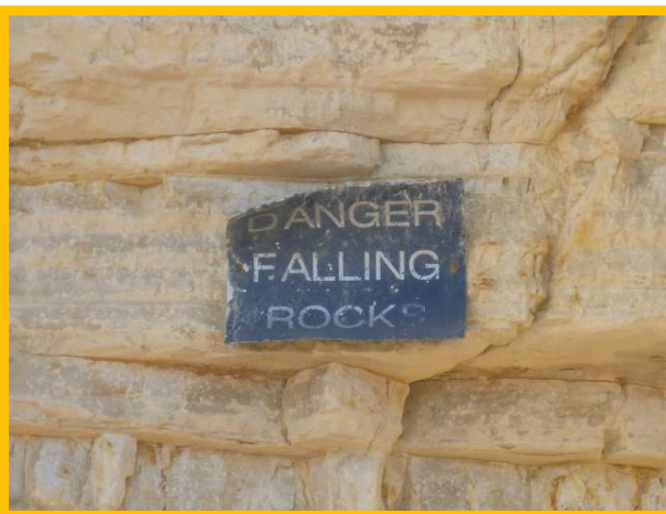
One small warning sign – bent condition (/0401C03)
