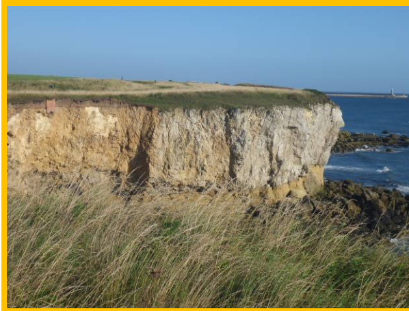
Undercutting at base of cliffs at Frenchman's Point (/0401C04)
