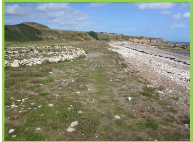
Backshore and slopes well protected by wide foreshore at northern section of Rifle Ranges (/0502C02)
