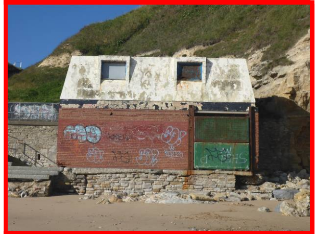
Undermining and voids at disused lifeguard station (/0401C01)
