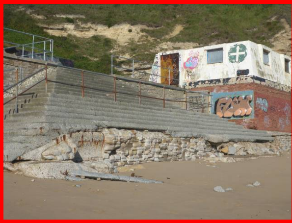
Undermining and voids at access steps (/0401C01)
