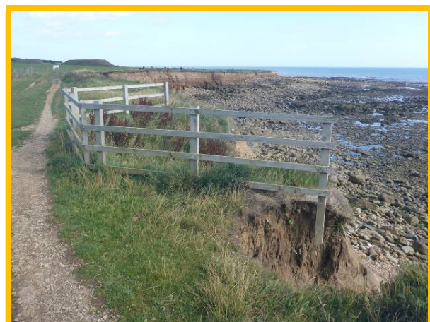
Repaired outfall – note loss of cliff top around fence post (/0601C02)
