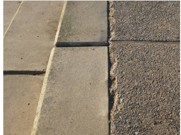
Minor abrasion at interface between stepped apron and promenade (/0102C02)
